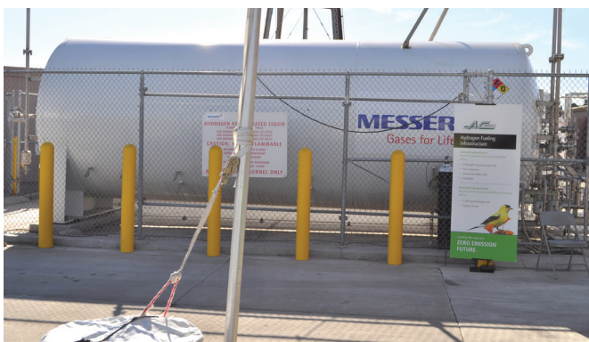
The planned hydrogen fueling infrastructure at D-6 is set to support up to 100 hydrogen fuel cell buses.
