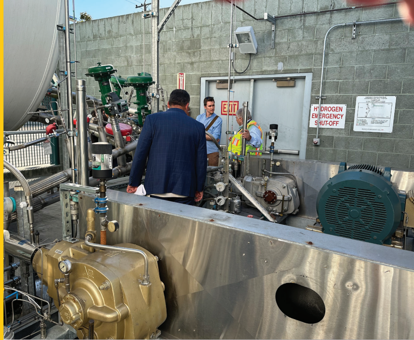
COO Salvador Llamas and Capital Projects Director Joe Callaway show Huls the mechanical operations behind D2's successful hydrogen facility.
