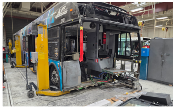
A bionic rebuild of the forward chassis structure included structural fabrication and welding, floor reconstruction, entry door replacement and alignment, and restoration of the wheelchair ramp.
