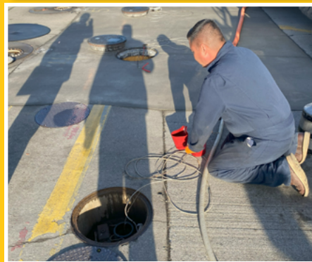
The above-ground storage tank was just one of many compliance areas where the District recorded zero environmental violations.
